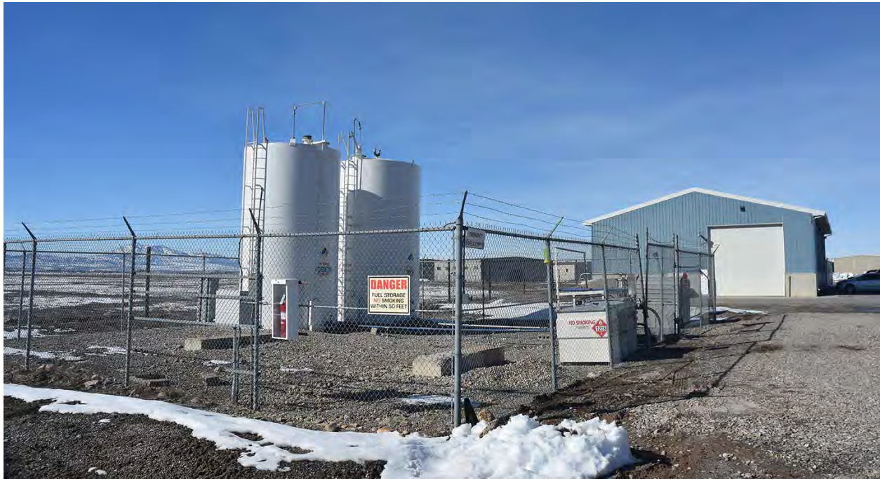
Figure 14: The LCCA fuel farm was installed in 1969. It is too small and functionally obsolete. It does not comply with modern Part 139 fuel farm standards.
